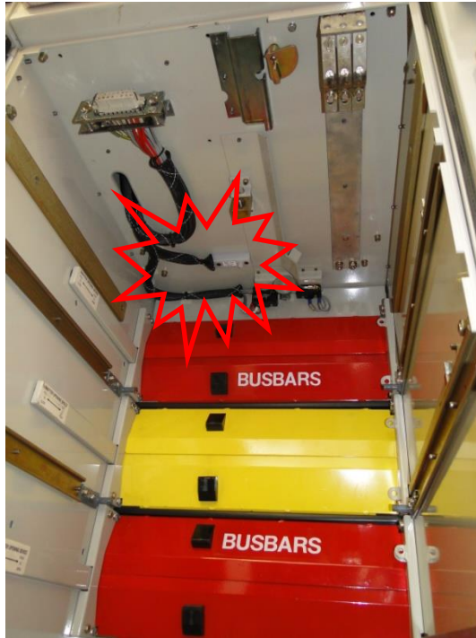
Sensor placement inside CB racking chamber
