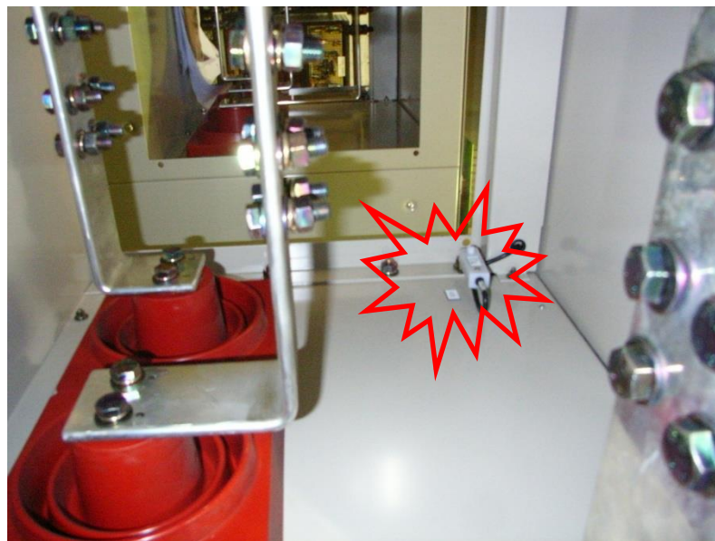
Sensor placement inside busbar chamber
